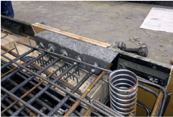
Fig. 3: Lateral view of the connections of socket bars on a disposable recess body
