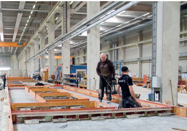
Integrating window and door recesses in the formwork with the aid of a MultiForm formwork support and MagFly AP
