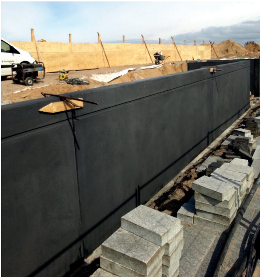
Anthracite-coloured flood protection wall in Heiligenhafen
