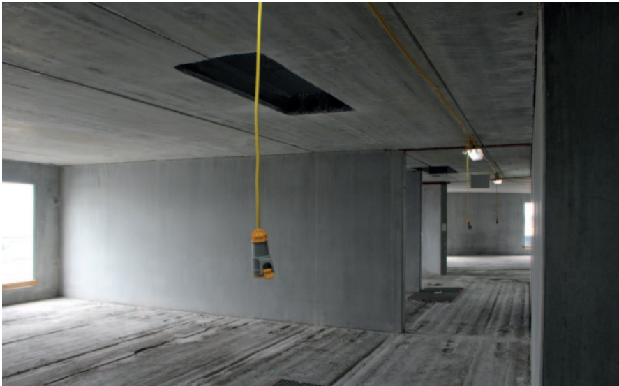
The complete hotel was originally to have been built using the cast-in-situ method. Now 12 storeys will be built exclusively with precast concrete elements.
