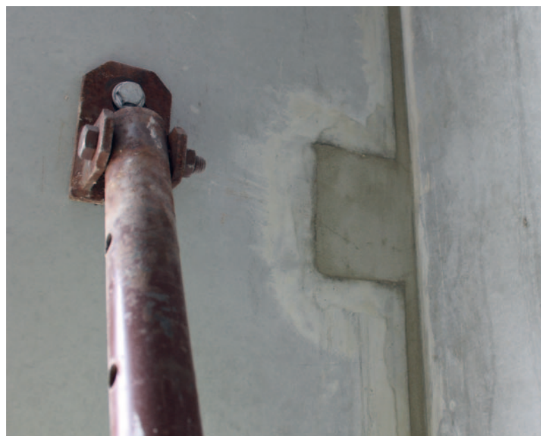
Once the precast concrete elements have been tensioned, the recesses can be sealed with grout.
