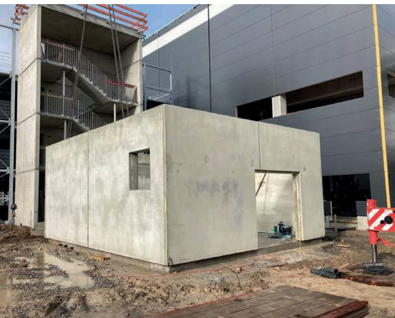
Sprinkler control centre fully assembled
