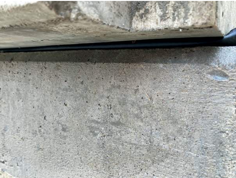
RubberElast instalada y comprimida
