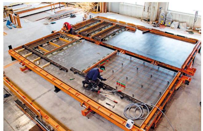
Fig. 7: View from the side catwalk of the battery mould down to the two work stations with the butterfly formwork lying folded out – on the right-hand panel of the completely visible butterfly formwork, the shuttering for three columns for the interior of a building is visible.
