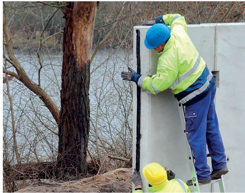
RubberElast® at the flood protection wall in Wittenberge
