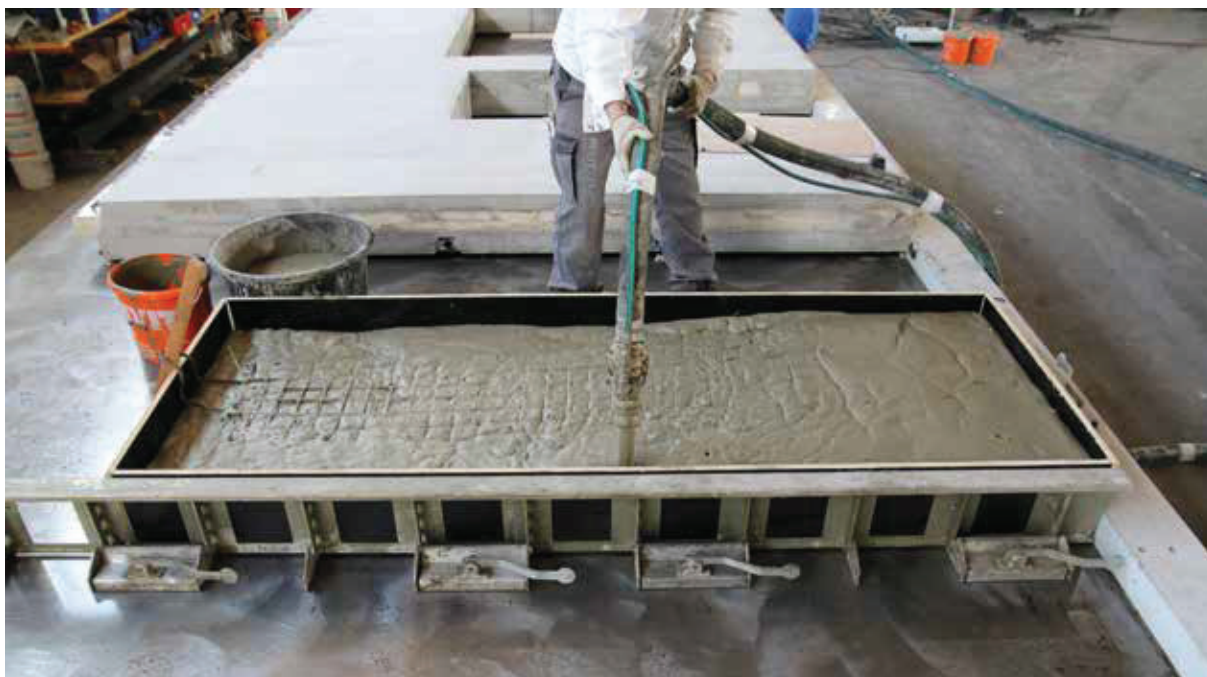
Figure 3: Horizontal production of a foamed-concrete wall: the wall has a thickness of 25 cm and serves for determining reference values for the wall produced in upright position
